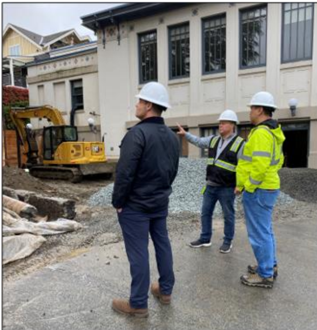
The Library team assess progress on the Green Lake Branch seismic retrofit project.
